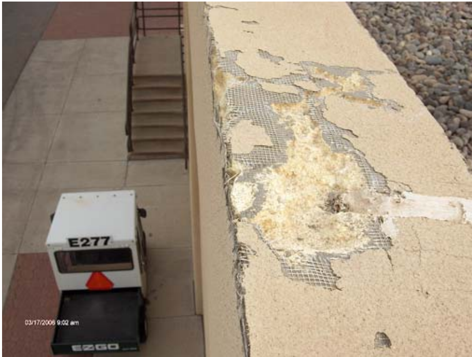
Figure A-1: Example of Typical Damaged Parapet
