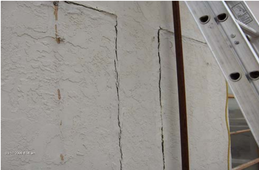
Figures A-3, A-4: Typical Examples of Structural Cracking on Multi-Story Building
