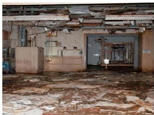
Advanced degradation due to roof failures and water intrusion. (2013)
