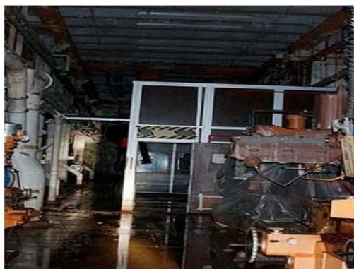
Facility condition and degradation, including standing water and contaminated equipment. (2013)
