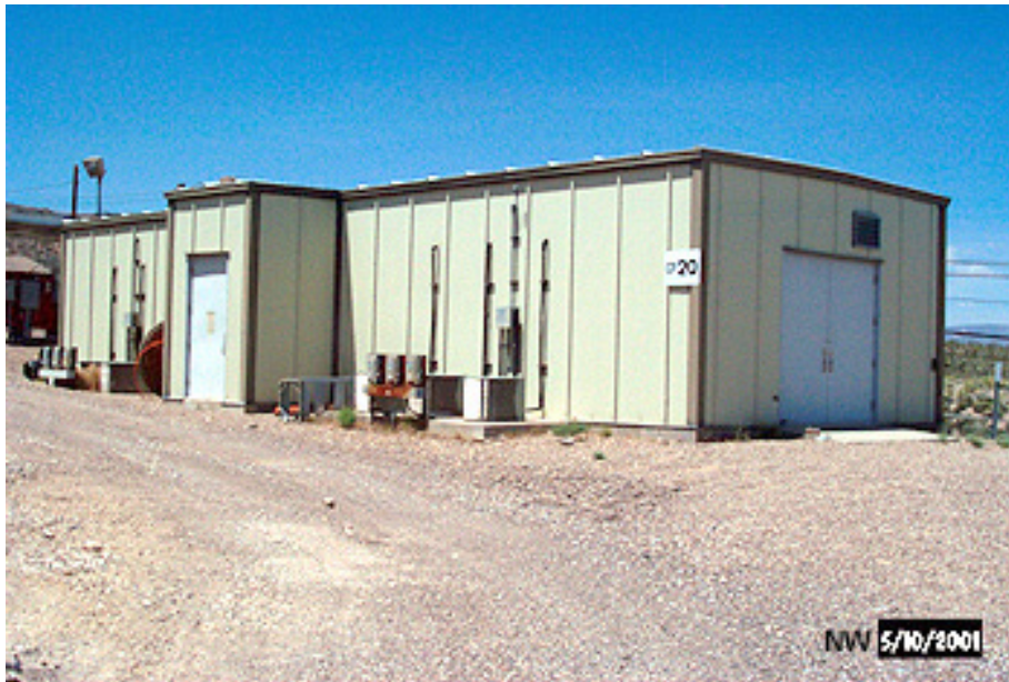
Figure A.8-6 — CP-20 is an ideal facility for housing the electronics for the Flight Test Program
