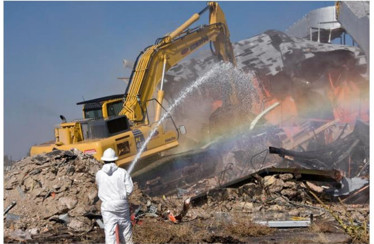
A worker suppresses dust during the final demolition stages of the historic DP West site, located at Los Alamos National Laboratory's (LANL) Technical Area 21.
